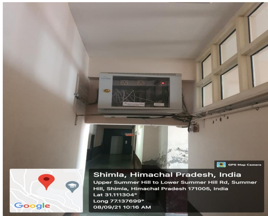
Networking Switch Rack
