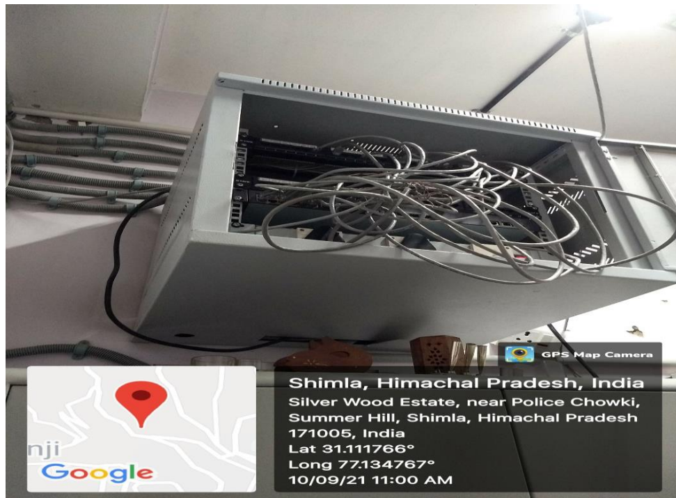
WI-FI Facility (2 ND Floor)
