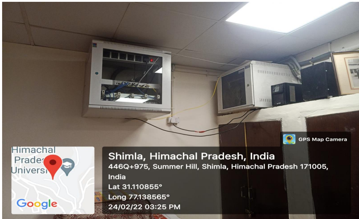
Internet Switch for office computers
